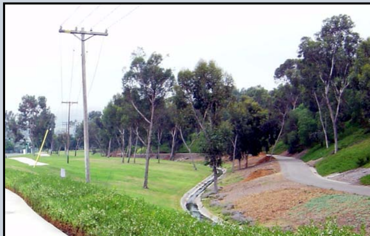
Removal of concrete v-ditch and restoration of low flow channel and flood plain in the Middle Reach of Upper Sulphur Creek.
