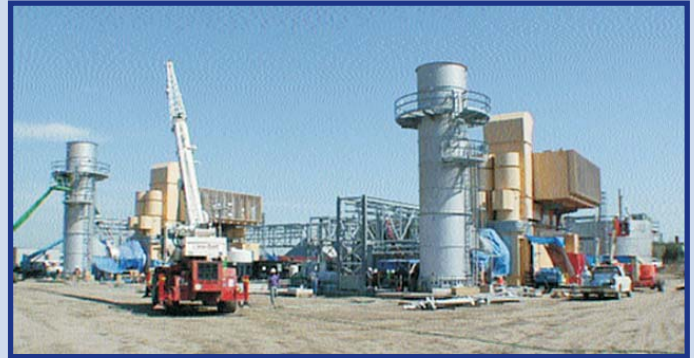
Aspen is providing staff support to the California Energy Commission for its permitting process and construction monitoring
